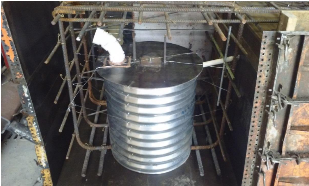
Figure 44. Side view of CMP void
