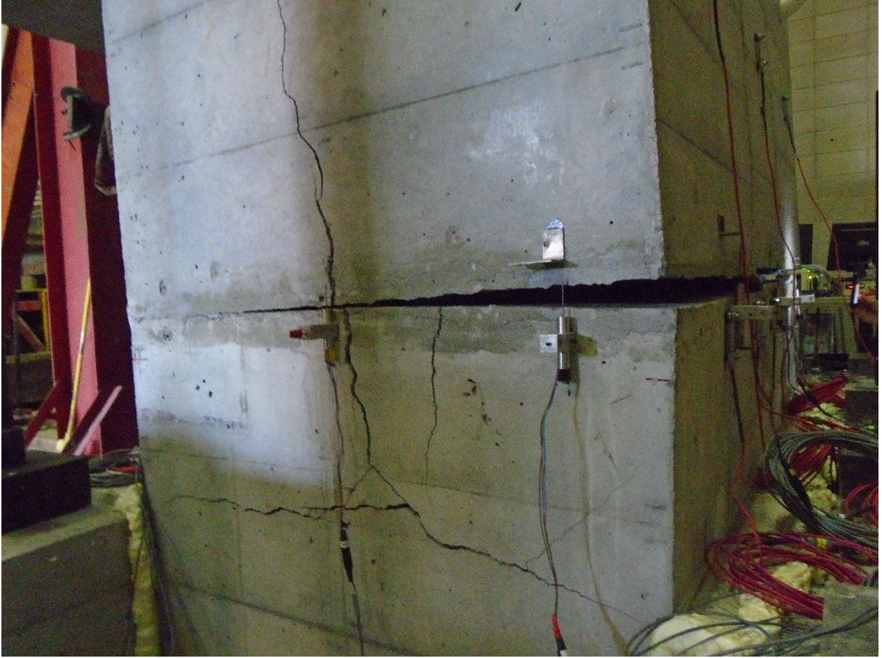
Figure 77. Pile coupler damaged west side
