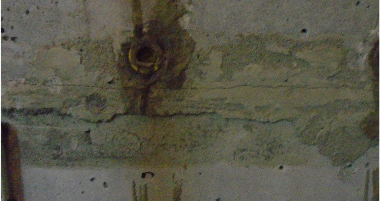
Figure 73. Crack between grout bed and diaphragm
