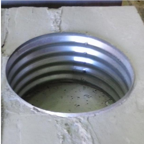
Figure 39. CMP void in pile cap
